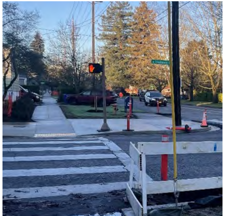
SW Corner of N Willis Boulevard & N Chautauqua Boulevard before (top) and after (bottom) stop improvements with sidewalk infill and new curb ramps.
