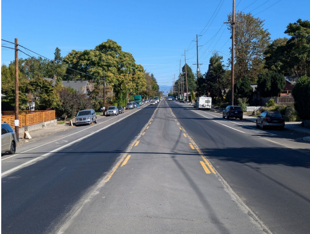
Figure 1 – Looking east on NE Killingsworth Street near 57th Avenue showing completed pavement grind and inlay of vehicle travel lanes.
