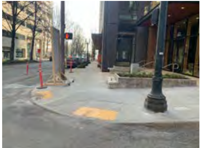
A developer rebuilt the corner of SW 2nd & SW Columbia through a permit as a part of their construction project. Source: PBOT.
