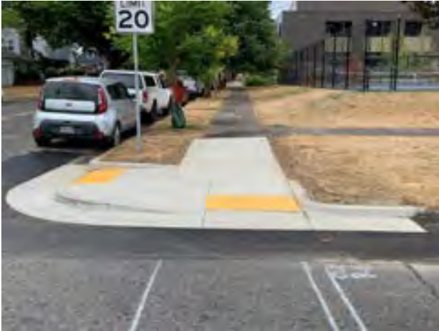
The corner of N Smith & N Ida was rebuilt as a part of a capital project. Source: PBOT.
