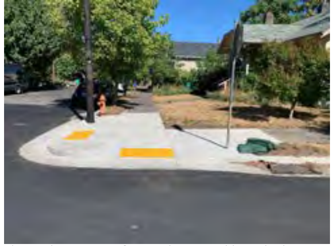
This is the corner of SE 17th & Brooklyn which was rebuilt as part of a PBOT maintenance project. Source: PBOT.
