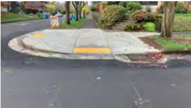
This is the corner of NE 30th & Klickitat where the corner which was a Ramps by Request location and delivered by a curb ramp only project. Source: PBOT.
