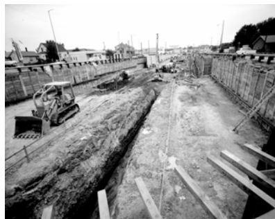
Construction of Powell under crossing at 17 th Ave, 1974. City of Portland Archives
